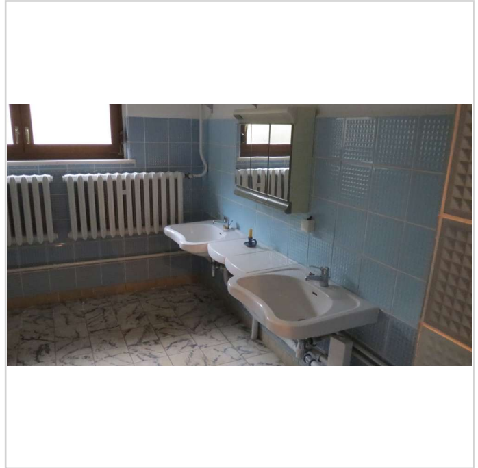
UG- BAD- WT- Anlage
